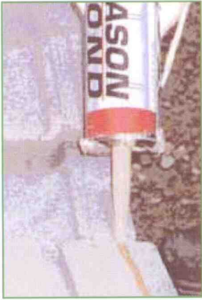
Mason Bond™ applied to vertical surface of the masonry block before it is set in place.
