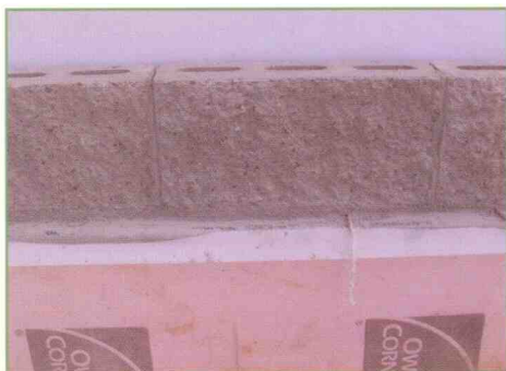
After seating the first course on a mortar bed, Mason Bond™ was used to secure the remaining 13,000 concrete masonry blocks.
