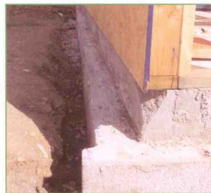
Despite having no masonry experience, students were able to lay over 700 blocks in just five hours of class time, and were able to backfill the walls the very next day!
