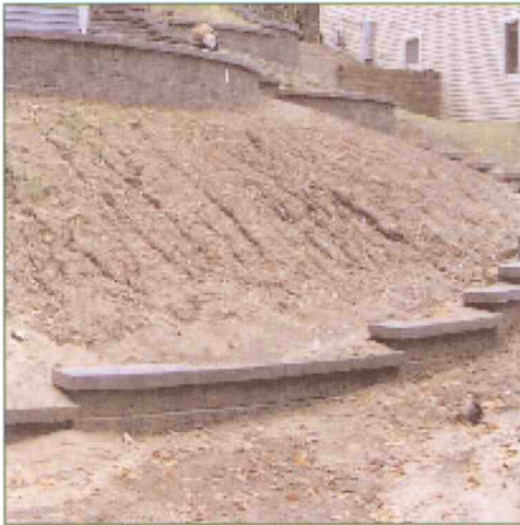
A rain storm washed some of the top soil down the slope, but the retaining wall built with Mason Bond™ stayed in place.
