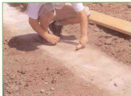
CMUs were adhered directly to a floating foundation using Mason Bond™ from ITW TACC.
