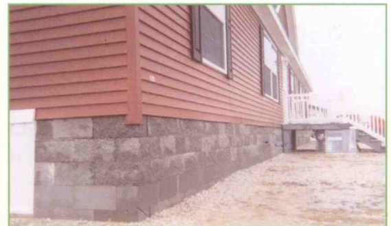
The finished skirting includes split-face architectural blocks adhered with ITW TACC's Mason Bond®.
